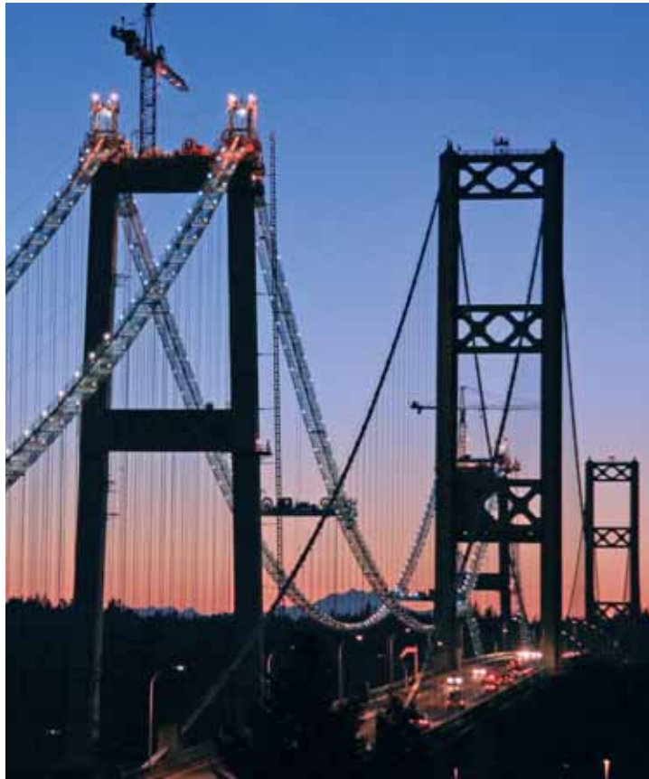
THE NIGHT'S ALRIGHT Construction on the new Tacoma Narrows Bridge in Tacoma, Wash., continues into the night.
